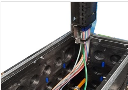
BPEO ECAM with Gasstop Installed on Mobile Bracket (MOBRA) in Manhole
